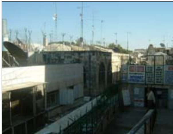
Fig. 5-26: The influence of new added steel windows in Jerusalem Old City (researcher).
