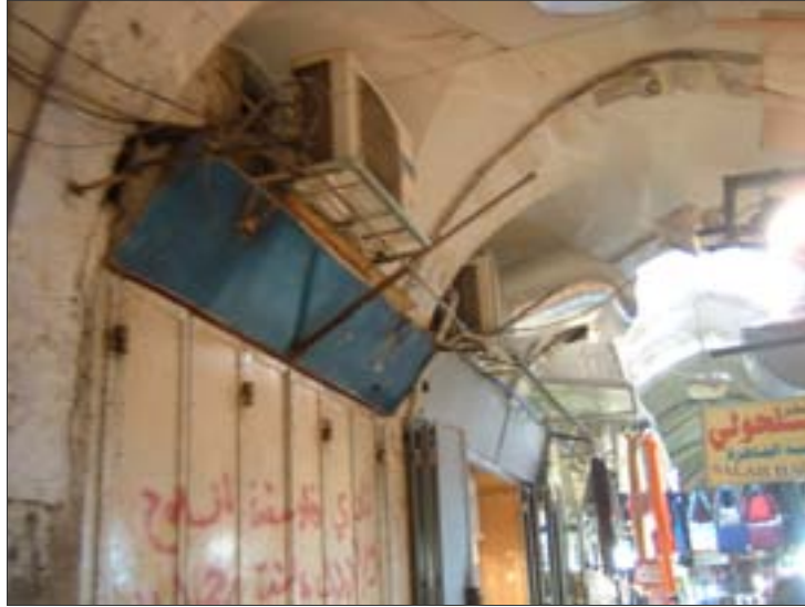
Fig. 5-25: The Added signs, ducts, and air conditioning, which influence the whole city image in Jerusalem Old City (researcher).
